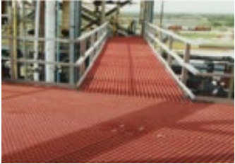
Stairways, grating, handrails, elevated walkways throughout the facility
