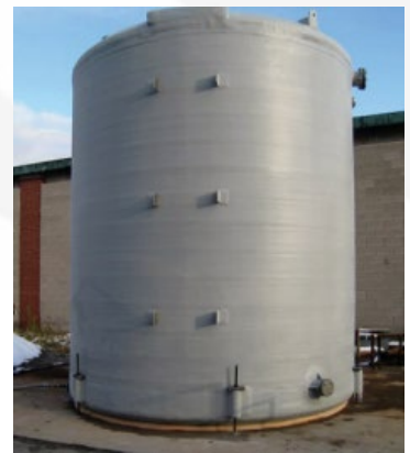
Storage Tanks - NaOCl, HCl, NaOH
