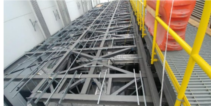
Mechanical support mezzanine
