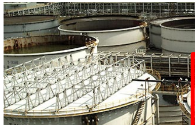
Covers, scrubbers, ductwork near settling ponds
