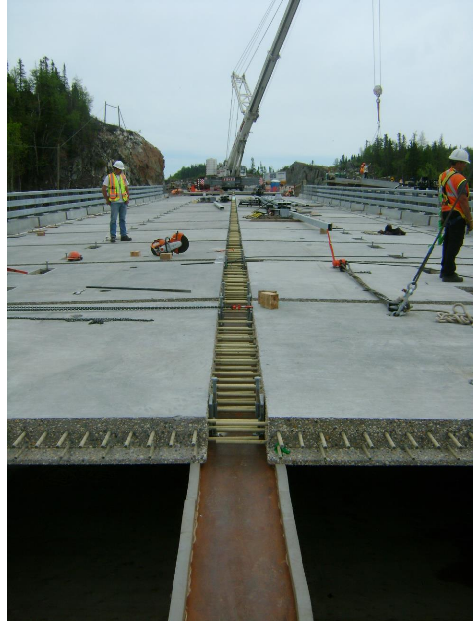
Steel River– MTO NW
