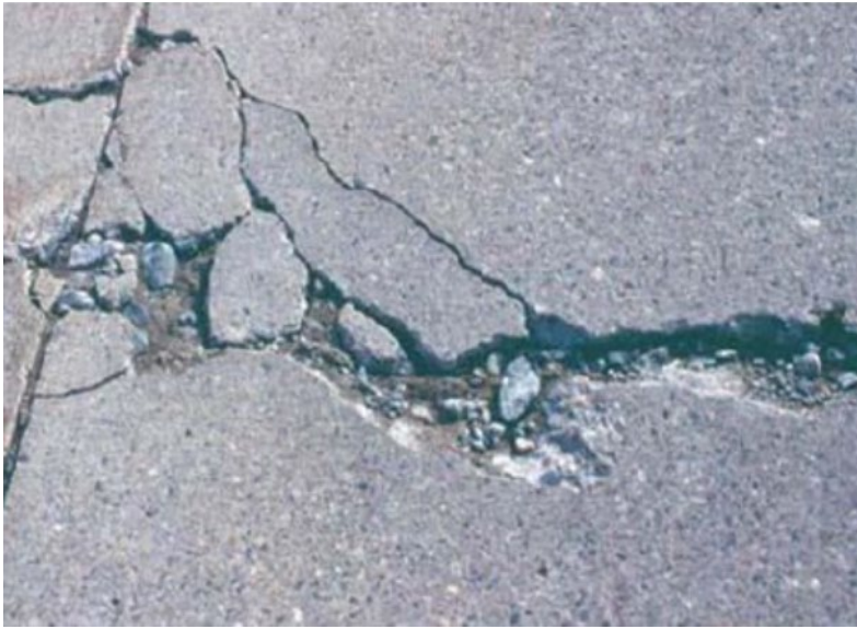
Freeze/thaw due to water ingress
