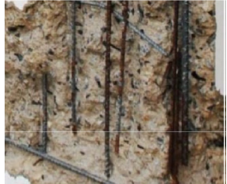
Chloride induced corrosion
