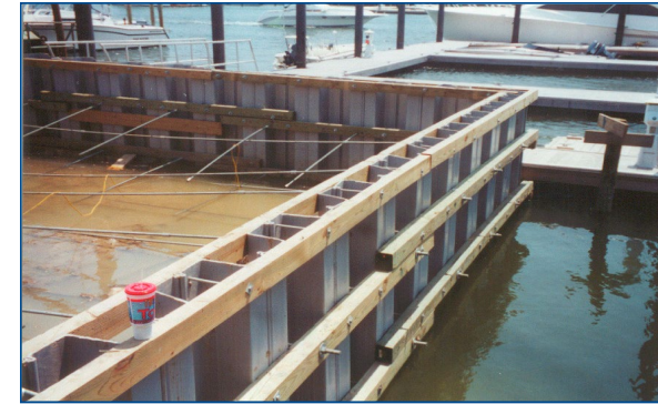
PVC deflects and requires additional walers
