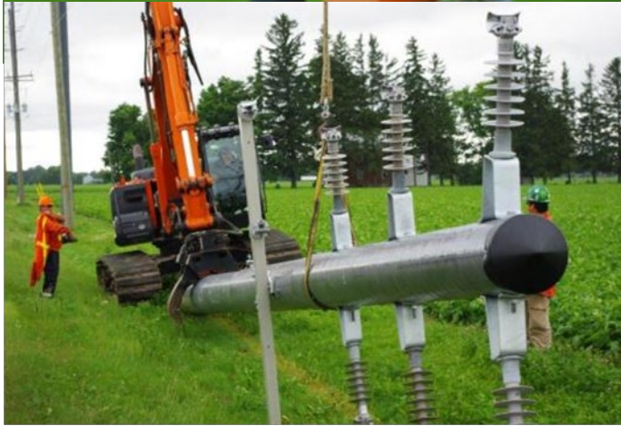
Grid Hardening after storm damage
