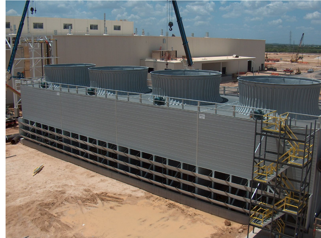
Photo of Cooling Tower Courtesy of Creative Composites Group
