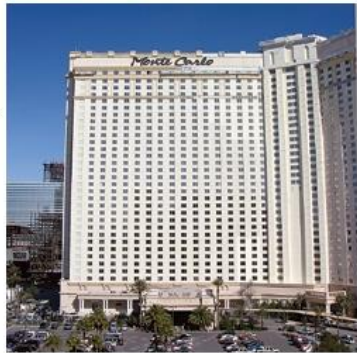
Fire damage to hotel was restricted to the upper facade, which has already been repaired (Bottom).
