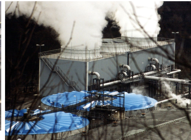
Cooling tower of pulp and paper mill; Source: Fiberline A/S
